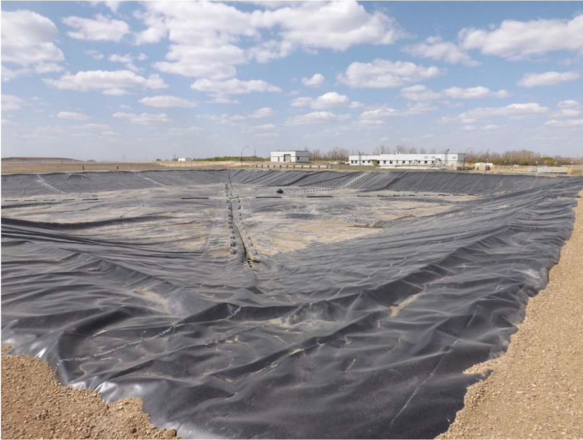
Figure 3: Lystek Storage Lagoon unfinished with Wastewater Treatment Plant in background.
